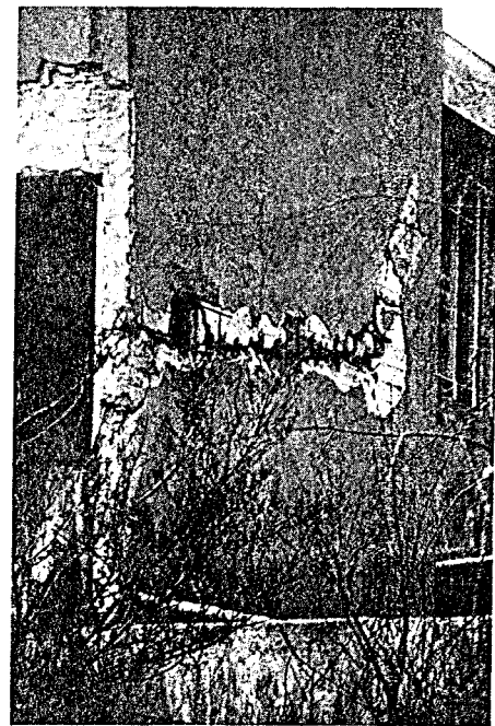
FIG. 33. Sliding shear in the shear wall of the Red Crescent Business Centre.
