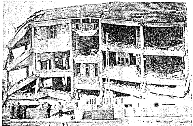
FIG. 16. Example of a reinforced concrete frame building with well-confined interior circular columns and poorly confined exterior square columns (courtesy of Profs. Ersoy and Tankut).
